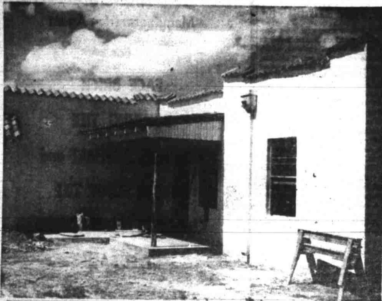
TILE COPING , metal window sashes are among modern features of this house under construction. (Photos by Jack M. Haynes)
