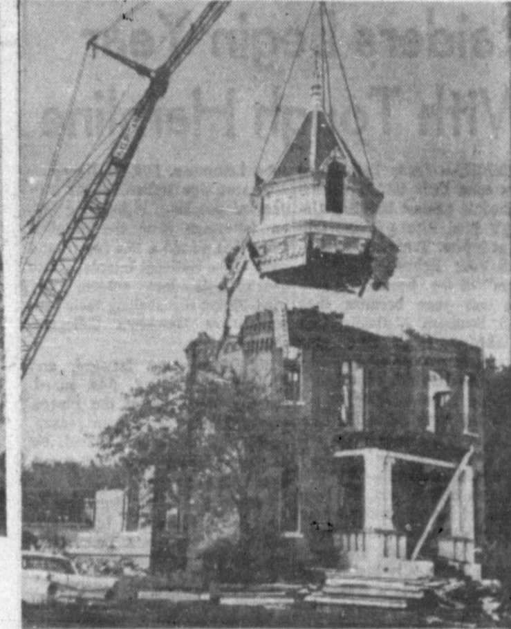
HEADING FOR OBLIVION —As a wrecking crew lifted the cupola from this old house in Dallas, Tex., it signalled the end of the two-story structure. But it meant the beginning of a new parking lot, more important in this age.
