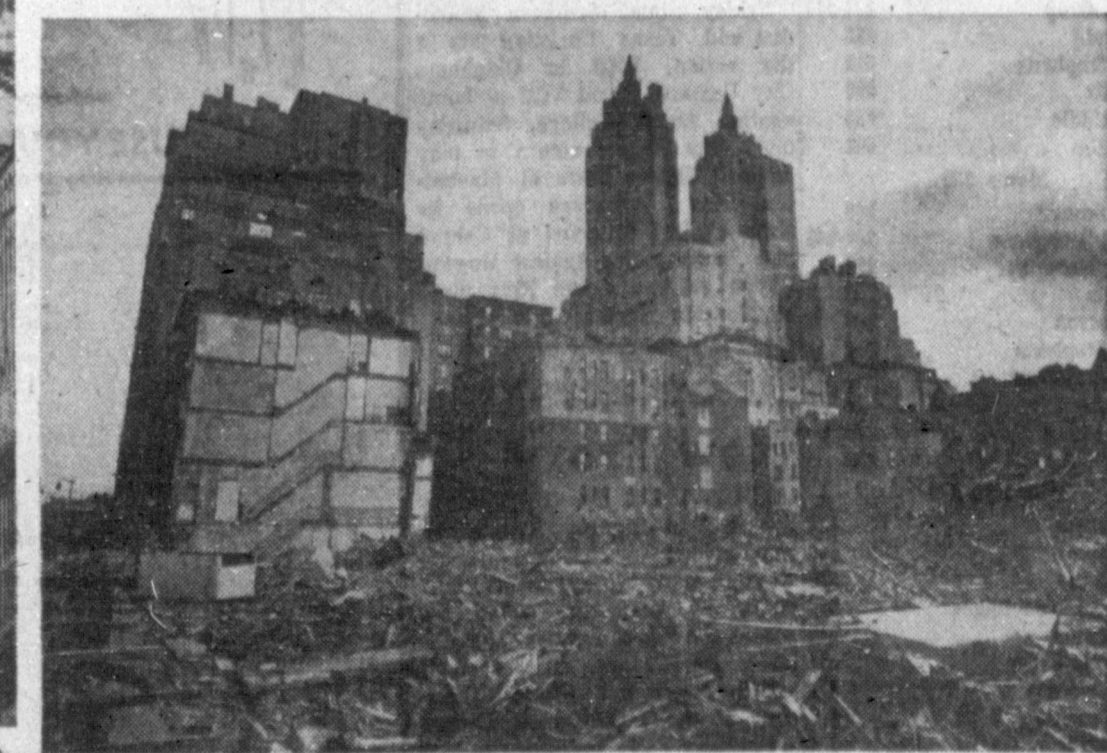
GOING UP AND DOWN —The soaring structures of the Manhattan skyline contrast with the mass of debris fronting them near Central Park. The building at left still has the imprint of stairways and windows of an adjoining structure that was torn down. It is part of a slum clearance project for a new public school on the West Side.
