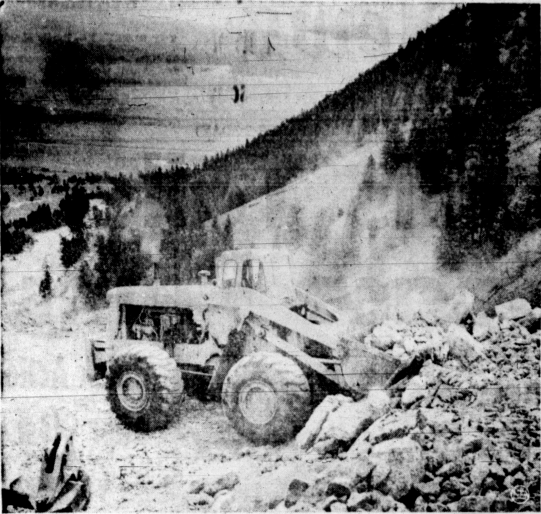
WORK IN EARTHQUAKE VALLEY —A tractor-shovel burrows through a mass of rock and dirt, part of about 43 million tons that were shifted in the Aug. 17 earthquake in Yellowstone National Park. U.S. Army engineers are building a spillway through a giant dam formed across the Madison River when the slide occurred. The impounded waters must be released to avert another disaster. The slide may also hold bodies of victims unlisted in the known toll of nine dead.
