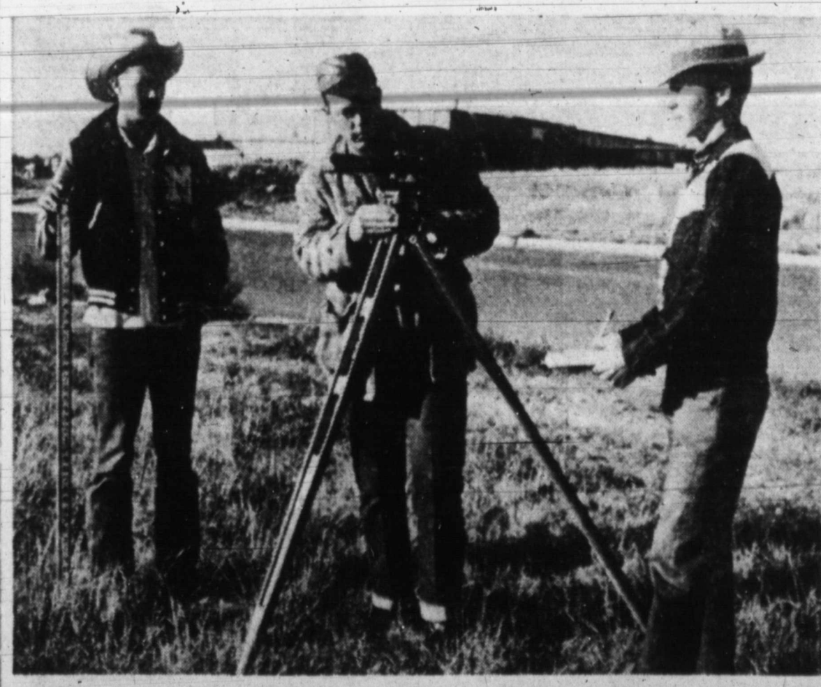
SEWER LINE FIELD CREW — One of the larger city sewer line projects in recent years will get underway Nov. 1 in Pampa when the Walter D. Bellamy Co. of Monahan begins laying five miles of line. The project, costing taxpayers $147,862, will take four to five months to complete. Seen above setting grade stakes for the line is the field crew for Roberts, Merriman, Bowden and Isbell, from left, Frank Willard, Don Willard and Don Stafford. In the background is the Coronado Inn, one of several additions to be served by the new line. The line will extend from southeast Pampa to the disposal plant, with one arm extending across the hotel property. (Daily News Photo)
