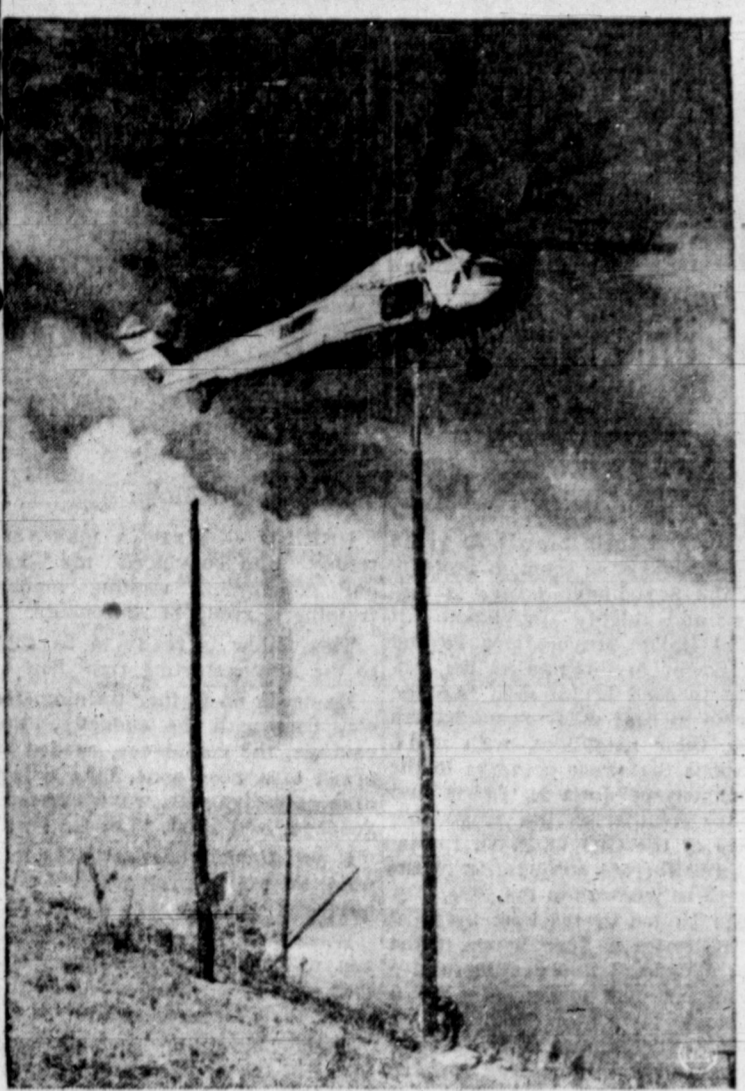
POLE VAULTER—As easily as sticking a candle in a birthday cake, a helicopter hovers over rough terrain on Puerto Rico to gently lower a two-ton power line pole into place. The Sikorsky S-58 aircraft is being used on a rural electrification project in remote sections of the island where there are no roads.
