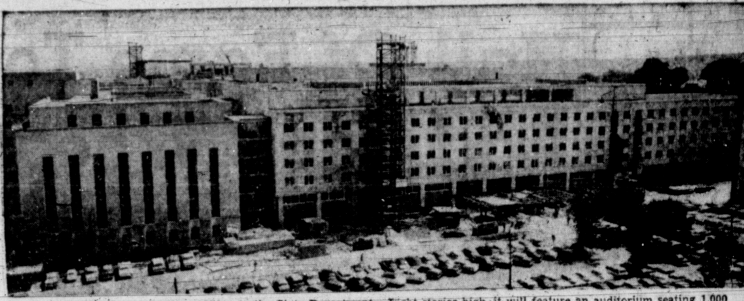
MAMMOTH ADDITION —Addition to the State Department Building in Washington, right, is three times the size of the present building, left. The completed headquarters will be second in size only to the Pentagon in the nation's capital. Eight stories high, it will feature an auditorium seating 1,000 and basement parking for 800 cars. It will provide for 8,000 employees and enable the State Department to gather under one roof all its workers who are now in 29 separate buildings.
