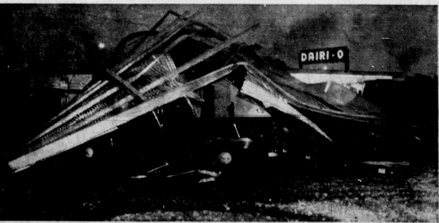
McLEAN STORM DAMAGE Residents of McLean and nearby Heald, slashed late Monday by heavy rains and a tornado respectively, were still counting their property damage today. Pictured here is the toppled and bent tin canopy of the Highway 66 Dairy-O, owned by Bob Taylor, in McLean. At left in background is an overturned trailer house. McLean received four inches of rain during the Monday storm.
