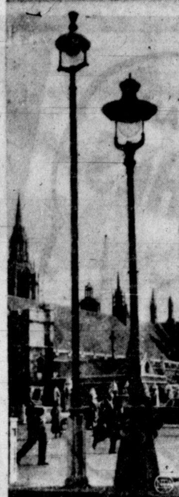
SIDE BY SIDE —The old and the new in London street lighting stand next to one another. Workers installed the new electric lamp before removing the old-fashioned gas lamp alongside. New lamp is at left.
