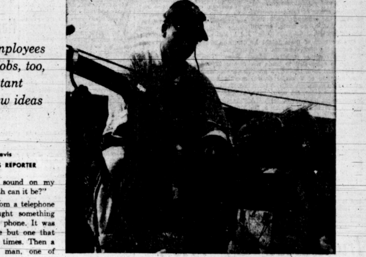
NEW TESTING DEVICE identifies wires in telephone cable twice as fast as before, cuts down customer complaints of noise. Determining which wire is which is necessary in repairing cable damage and hooking up phones. Cable Splicer Charles Thone, above, shows how the device works.
