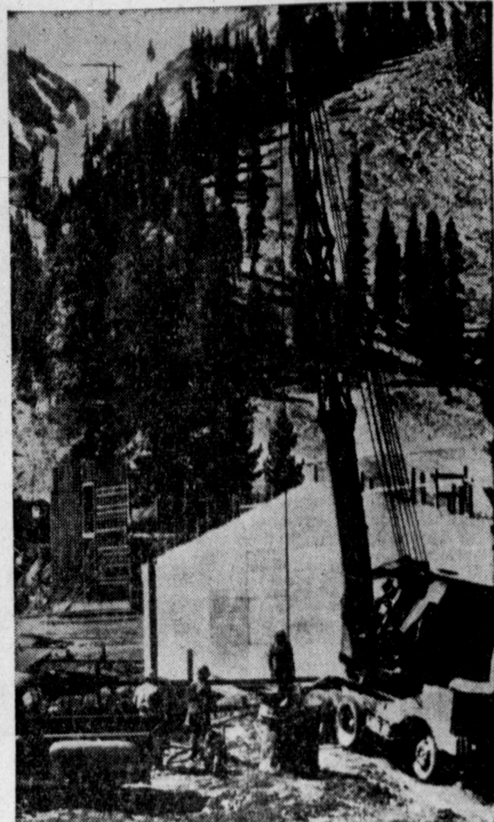
PREPARING FOR OLYMPICS —Construction is moving rapidly at Squaw Valley, Calif., where the VIIIth Olympic Winter Games will be held in 1960. Here, workmen prepare to pour concrete inside huge wooden form which shapes fire wall of the press building for the games. Papoose Peak and KT-22, where slalom, giant slalom and women's downhill ski races will be run, rise in the background. Work is well ahead of schedule.
