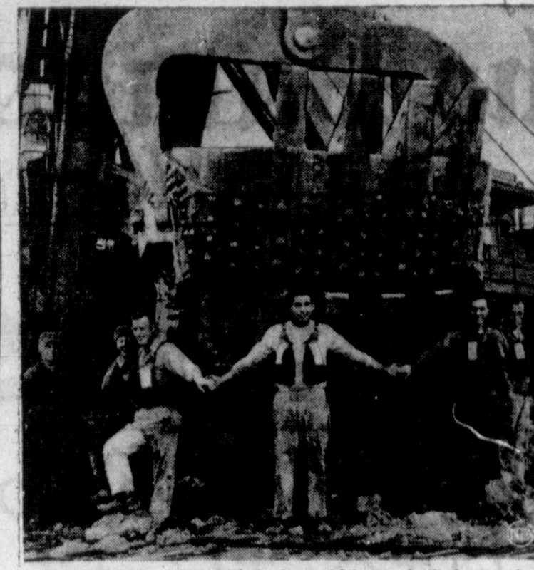
BIG DIPPER —This huge dredge, which was built for use in the Panama Canal, is scooping out a deeper channel in the Detroit River near Detroit, Mich., in preparation for the St. Lawrence Seaway. Crew members of the dredge link hands to demonstrate the size of its 22-ton bucket, which can gobble up 15 cubic yards of river bottom in one bite.
