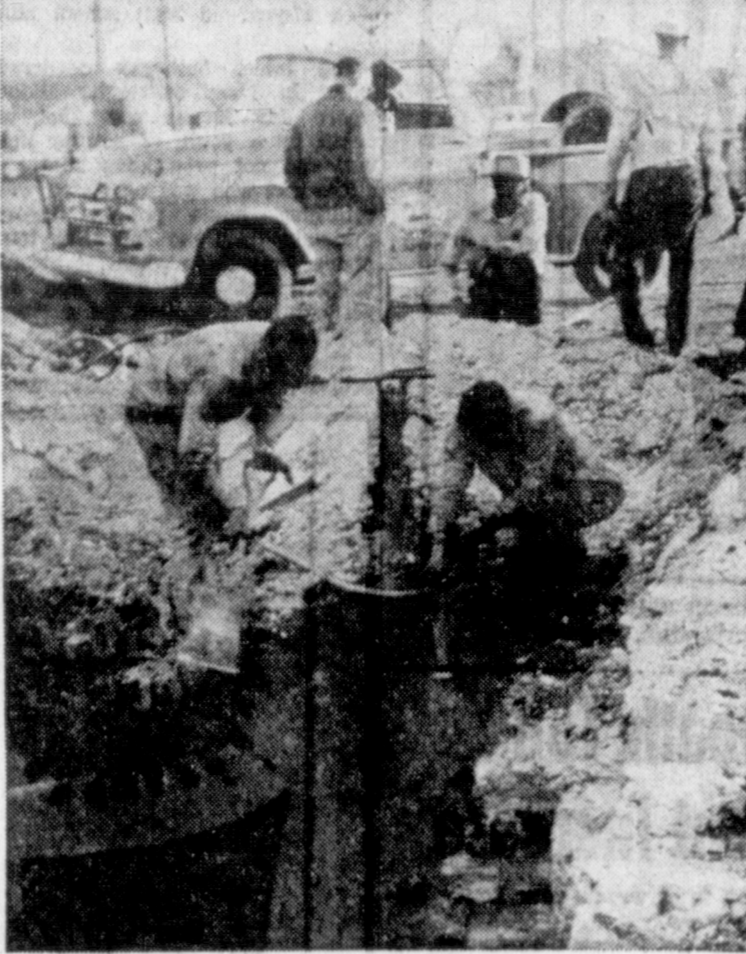
STORM SEWER CONSTRUCTION —Many of the intersections on Hobart street have been closed recently due to the construction of the storm sewer for the Hobart street underpass. Plans call for construction of the underpass to begin early next year and it should be opened for traffic by the end of the year. Workmen are shown above as they were digging around utility lines at the Hobart, Francis and Alcock intersection earlier in the month so that the storm sewer could cross the intersection. The long sought underpass will speed up traffic at the crossing and remove one of the main traffic hazards in the area. (News Photo)
