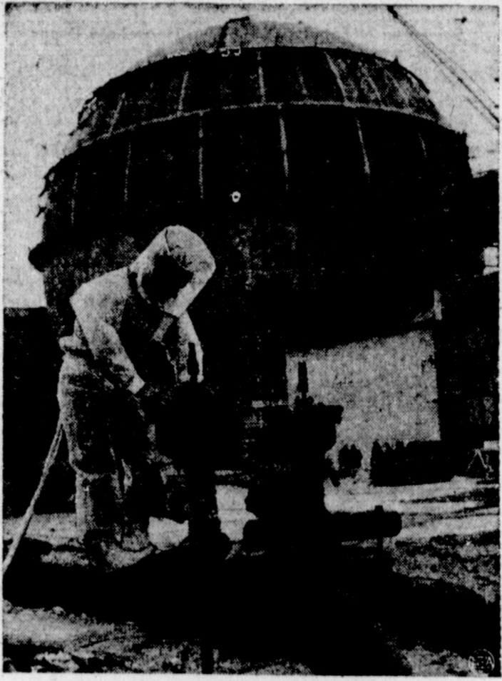
ATOMIC SAFETY —Protected by a lightweight suit which guards against radiation, a safety foreman shuts off a set of valves at the United Kingdom Atomic Energy installation in Dounreay, Scotland. The massive sphere, 135 feet in diameter, in background, is the housing for Britain's first big atomic breeder reactor. Designed as a source of cheap power, the reactor is expected to play a large part in ending Britain's fuel problems.
