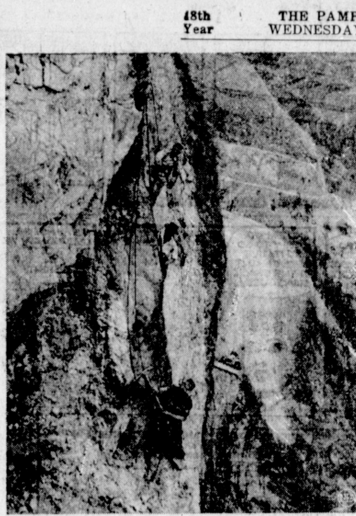
"WINDOW-WASHING" ROAD BUILDERS—A three-man crew of road builders use the U.S. window washer's technique as they "face up" the perpendicular side of a rock cliff at Caqueza, Colombia, on the new Villavieja-Bogota Highway. Smooth surfaces on the sides of the cliffs prevent torrential rains from causing erosion and landslides. The new road is 230 miles long and opens up the Colombian Llanos, a 250,000 mile "Texas-like" cattle country—virtually uninhabited. Starting at sea-level zero the road climbs to a chilly 12,000 feet and then goes down to 8,000 feet at Bogota.
