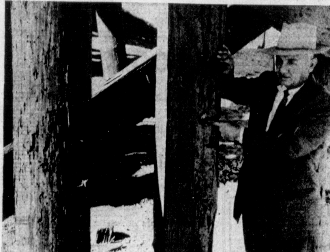
DAMAGED BY SHOOTERS — L. E. Sankey, division special agent for Santa Fe Railway Company, is shown pointing to one of the smaller holes in pilings in a bridge located on the "cow-line" which is located about one-half mile southeast of the Country Club, which was caused by persons discharging firearms into the bridge. Larger holes in other pilings had already been repaired. Charges will be filed against any person caught firing bullets into the structure. (News photo)
