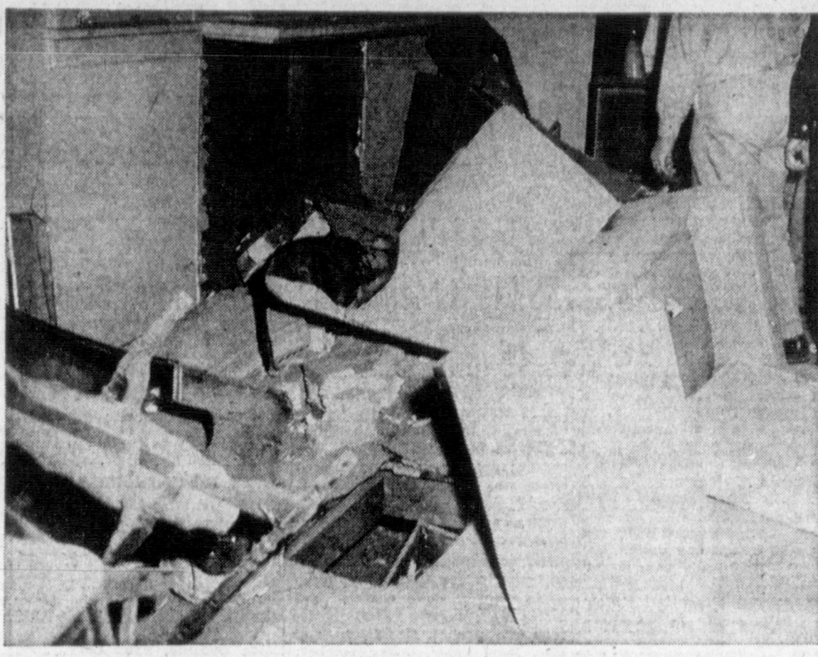
BLAST RIPPED HOUSE — Shown above is the interior of the living room of J. M. Gillpatrick at 718 N. Somerville after an explosion damaged the house about 5:45 p.m. yesterday. The explosion is believed to have been centered in the area of the floor furnace, the hole in the floor near the center of the picture. No one was in the house at the time. (News photo)
