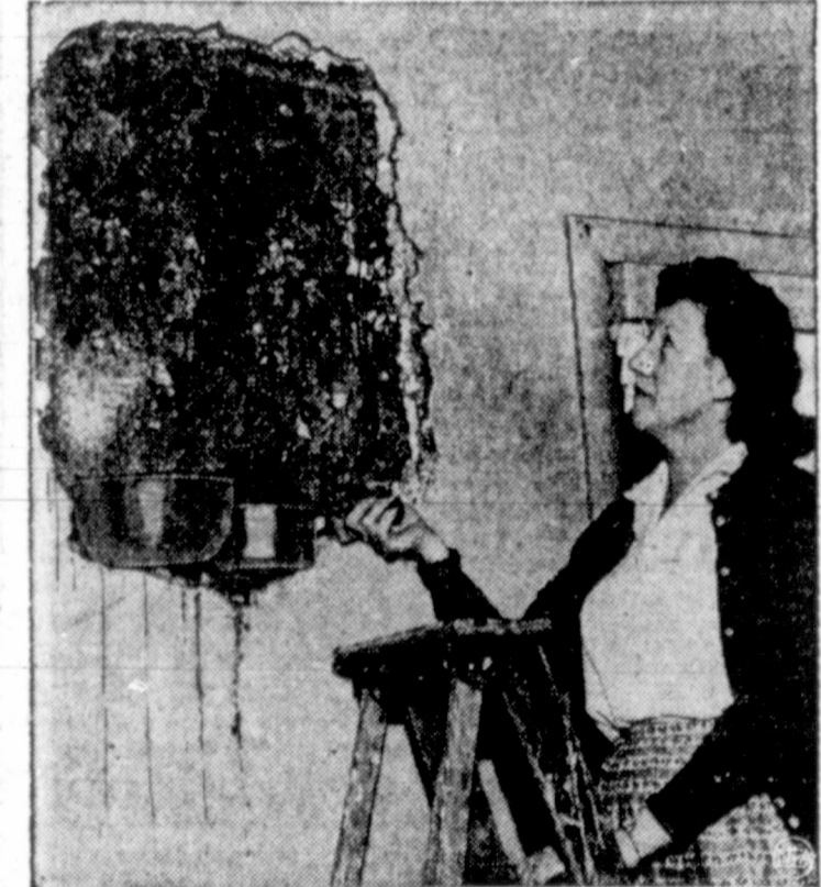
BEEZY IN THE KITCHEN —Mrs. Paul Tadrick, of Detroit, Mich., was bothered by an odd buzzing noise behind her kitchen wall, so hired a man to rip off the plaster. Above, she collects rent—two potsful of honey—from the honeycombed wall, where a swarm of bees had taken up residence.
