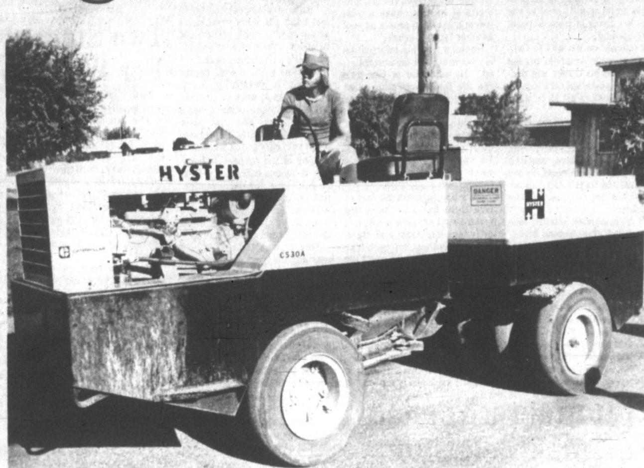
LAYING THINGS DOWN — Ken Prestidge of Lefors drives a pneumatic compactor during work on resurfacing of city streets in the Crestview Addition. Work started last week on
