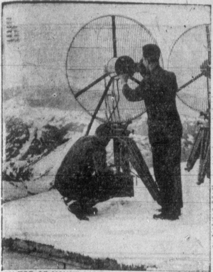
ON TOP OF MOUNT SANTIS—That's where these antennae are being installed by Swiss workmen. Switzerland's TV network is the highest in Europe, because the signals must be beamed over 8000-foot peaks of the Swiss Alps. This has greatly increased the cost and technical difficulty of establishing Switzerland's TV network.
