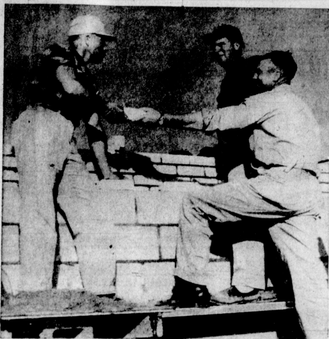
GOOD PROGRESS is being made on the McLean Clinic which is expected to be finished between Feb. 1-15. Work began last Nov. 15 on the 40 x 70 foot white brick structure which is rising rapidly with the laying of bricks. Shown above laying the bricks are McLean workmen Gene Swafford, C. H. Kelly and J. L. Crofford. Spears-McPherson are the local contractors for the work. C. P. Callahan, a member of the building committee, is helping to supervise the construction. (News Photo)
