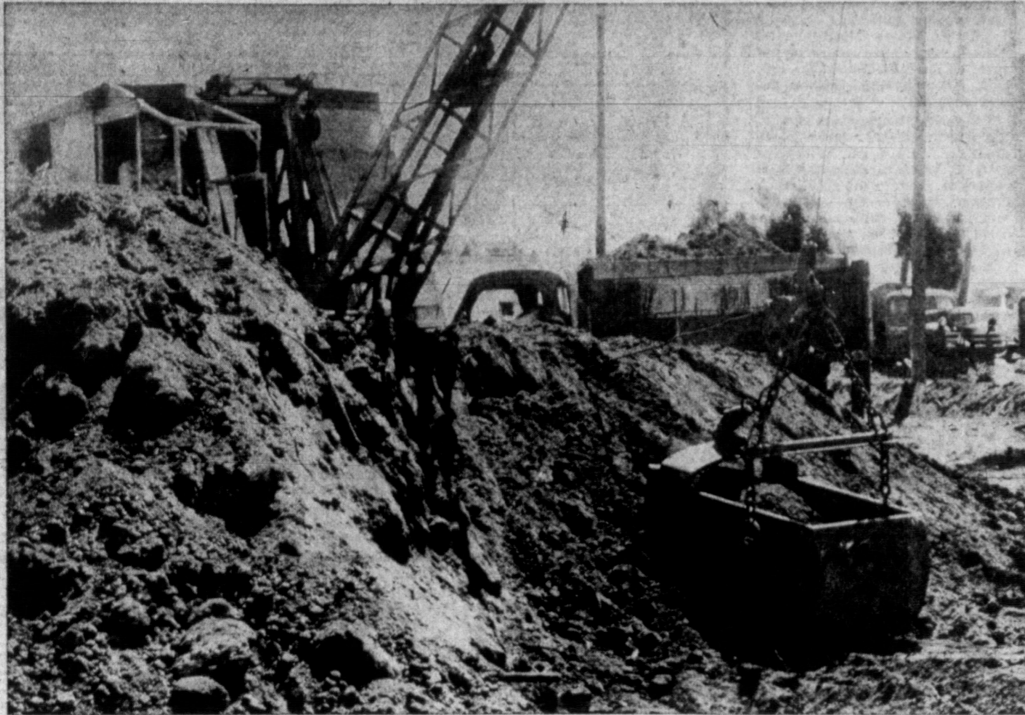
GROUNDWORK BEGINS — The ground work is under way at the corner of Purviance and Francis for the construction of Ideal's new supermarket. Shown above are a truck and shovel moving excess soil and leveling the site. The $125,000 store will be completed about January 1, according to the Blakemore Brothers, owners of Ideal Supermarkets. (News Photo)
