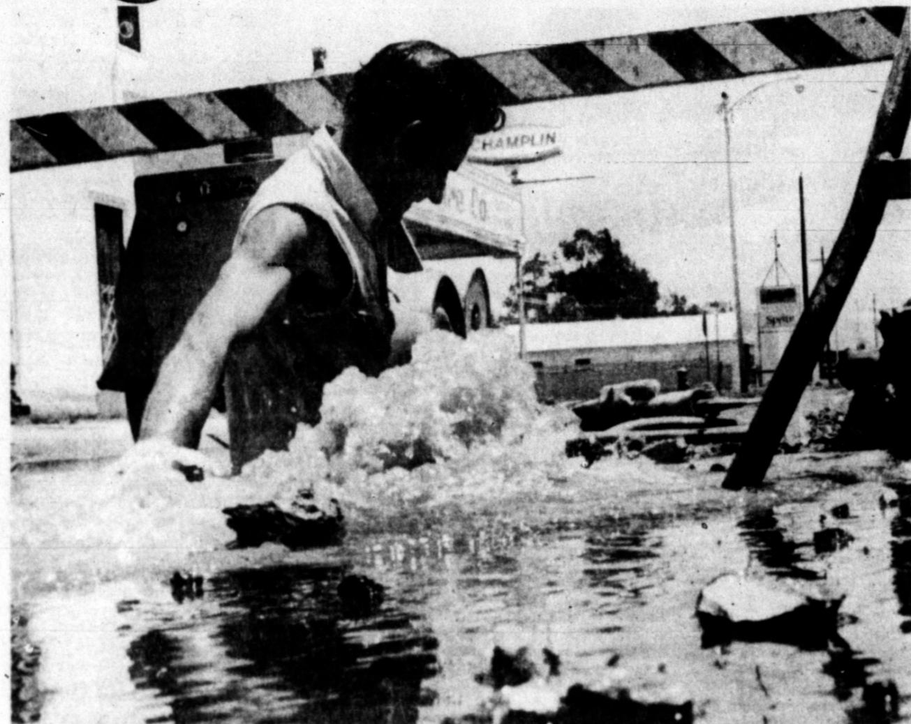
UP TO HIS WAIST — Dee Shackelford, city Water Department employe, lowers himself into a hole to repair a break in a two-inch water main. A band snapped on the pipe Tuesday afternoon in the 700 block of W. Foster, creating a small flood in the area until it was repaired yesterday evening. (Photo by Terry Hanna)
