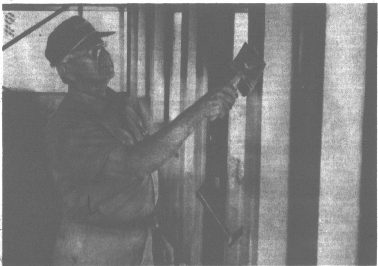
Doug DuBose works on the interior of the pro shop Thursday at the Pampa Public Golf Course. DuBose, a retired minister, is construction supervisor of the facility, which will include a snack bar, offices, utility room and cart barn. A work party is scheduled for
