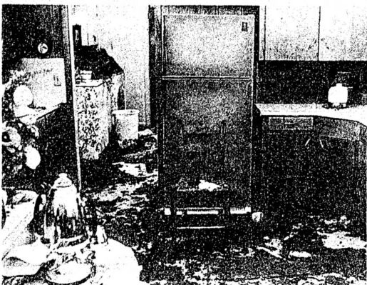
COVERED WITH DEBRIS — The kitchen of a house at the corner of Horsburgh and S. Talley Sts. in White Deer is covered with mud and other debris deposited by the tornado. The owners, Mr. and Mrs. C. E. Walker, were huddled up against the cabinets on the right. Walker received a cut on his hand.
