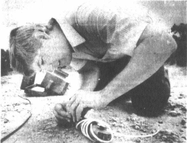
Howzer wires plastic explosives for demolition. (Staff photos by Duane A. Laverty)
