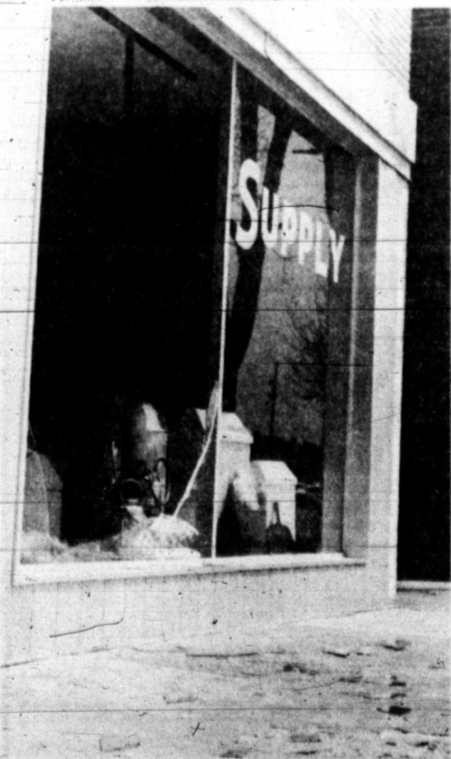
WIND DAMAGE — Gusts up to 90 miles an hour Thursday damaged various structures around the city. Examples of the damage include a plate glass window blown out, left, at Warner Janitor
