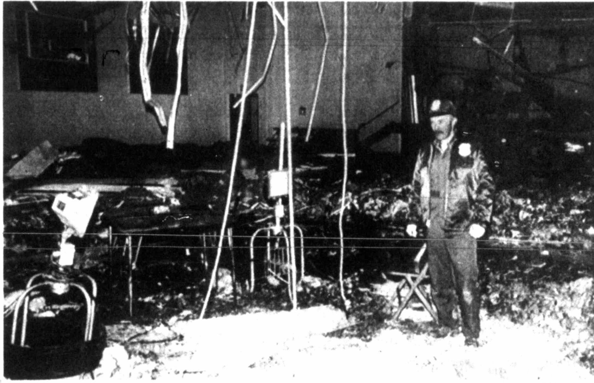
Investigator surveys church damage from blast.
