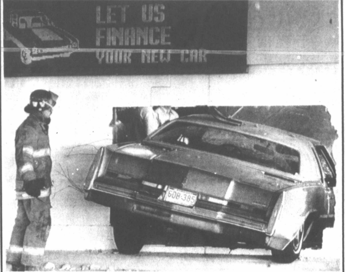
Charleston, W. Va., fireman Corbett Puffenbarger surveys the damage after an unidentified motorist drove his car through a wall of the drive-thru window at the United Bank in Charleston, Thursday. Police are investigating the incident.
