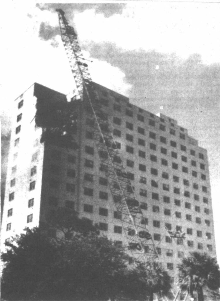
A wrecking ball knocks off an upper corner of the Shamrock Hilton Hotel in Houston. The razing could take five or six months, according to Texas Medical Center officials. The center bought the hotel and plans to build a research center on the site.
