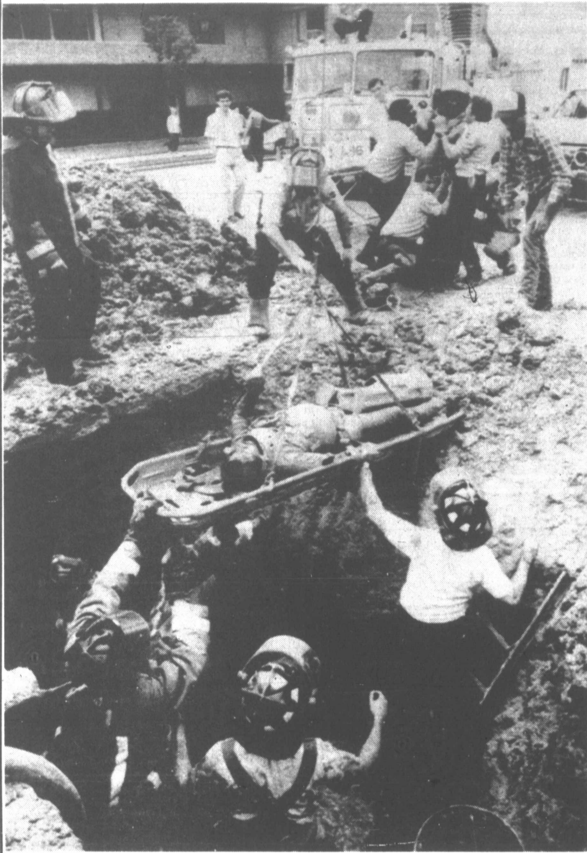
Construction worker Agustin Espirito is lifted by Houston firemen out of a street excavation in which he was working Friday. The damp walls had given way, causing a mudslide that trapped Espirito for about an hour. Espirito was listed in stable condition at a Houston hospital.
