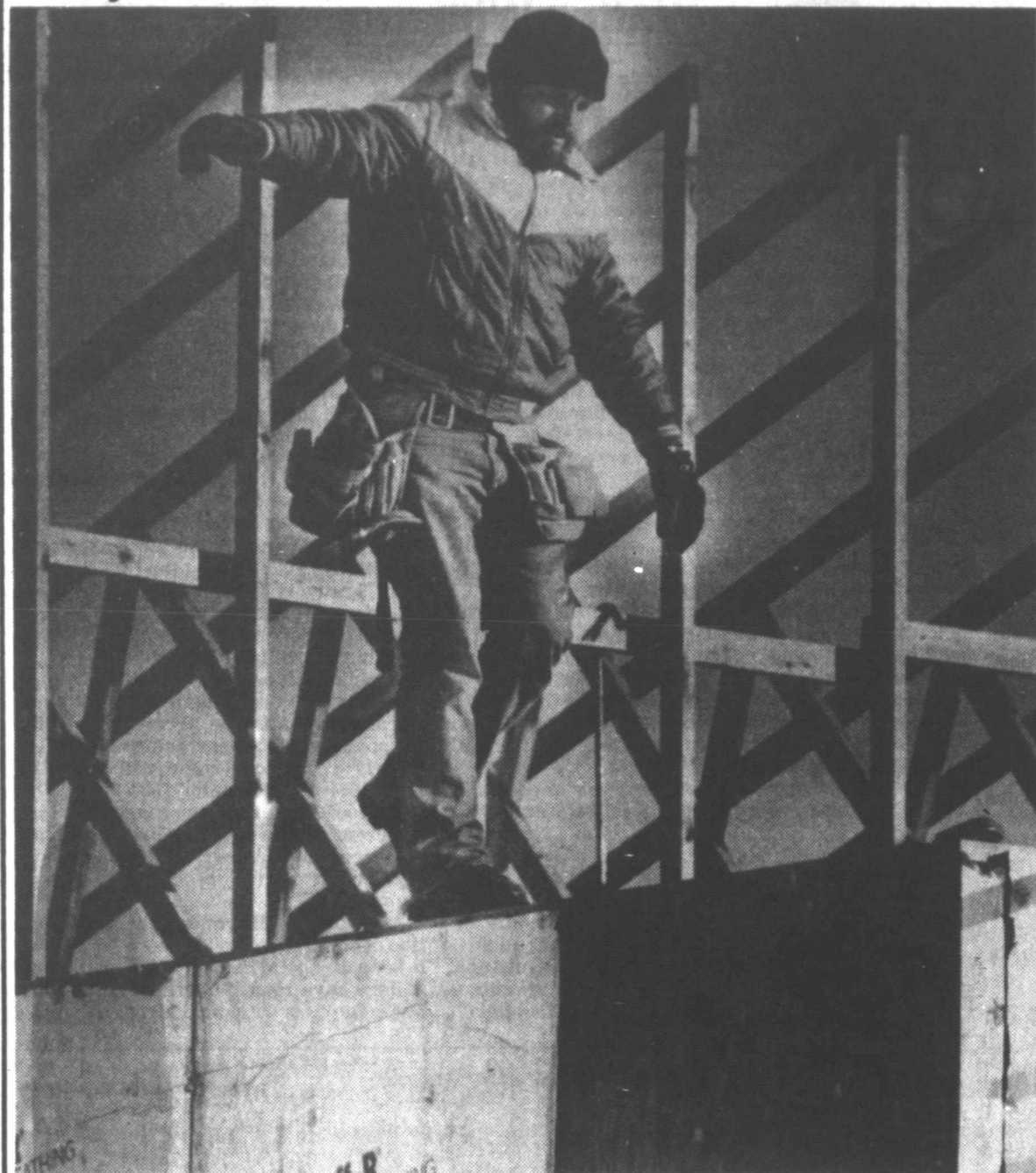
A construction worker steps carefully along an unfinished wall at the site of the Lakeside Apartments near the 2500 block of North Hobart. The worker got a break in the weather last week, but more cold temperatures were forecast for today. The forecast called for freezing drizzle or light snow and a high near 30. (Staff Photo by Duane A. Laverty)
