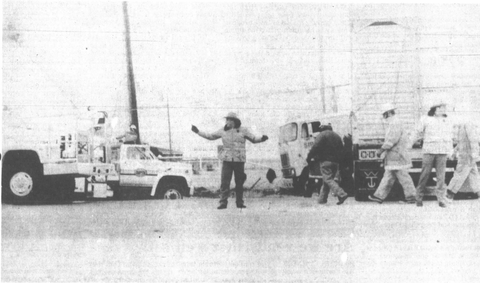
DPS units direct traffic while SPS units repair a transformer at scene of real accident on Hwy. 60.
