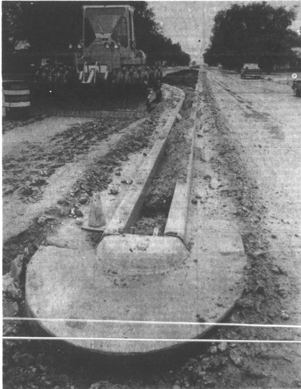
MEDIAN START—The much-discussed median on Somerville is beginning to take shape as reconstruction work on the street continues. (Staff photo by Terry Ford)
