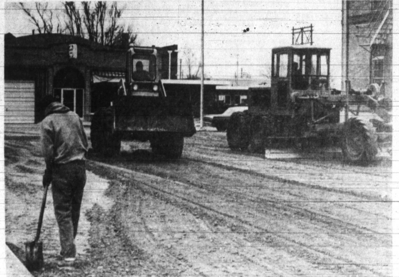
LAYING THINGS DOWN — Construction has begun on a new parking lot behind the Central Fire Station where the old water tower, torn down last summer, used to stand. From left are James Brown, using a shovel, and Raymond V. Jennings and Woody Hubbard, operating equipment to level the land. (Photo by Doug Abbott)
