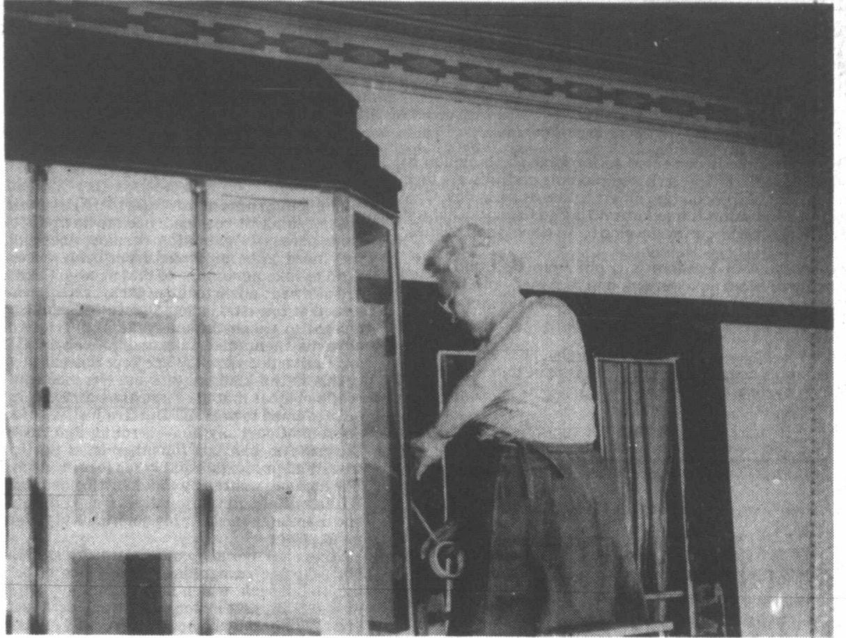
TRIM TAPING — Leta Mae Hess sticks tape on windows of the Avalon Theater Box office in preparation for painting as part of the downtown McLean facelift. (Photo by Cathy Spaulding)
