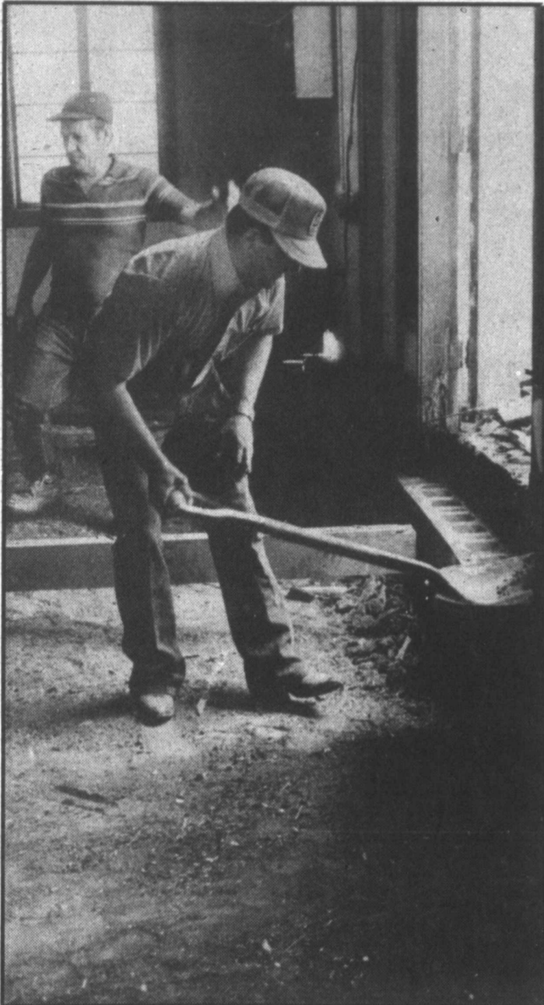
THE REV. LLOYD Burd, left, and McLean Assembly of God member Lee Brown clean the gutted front hall.
