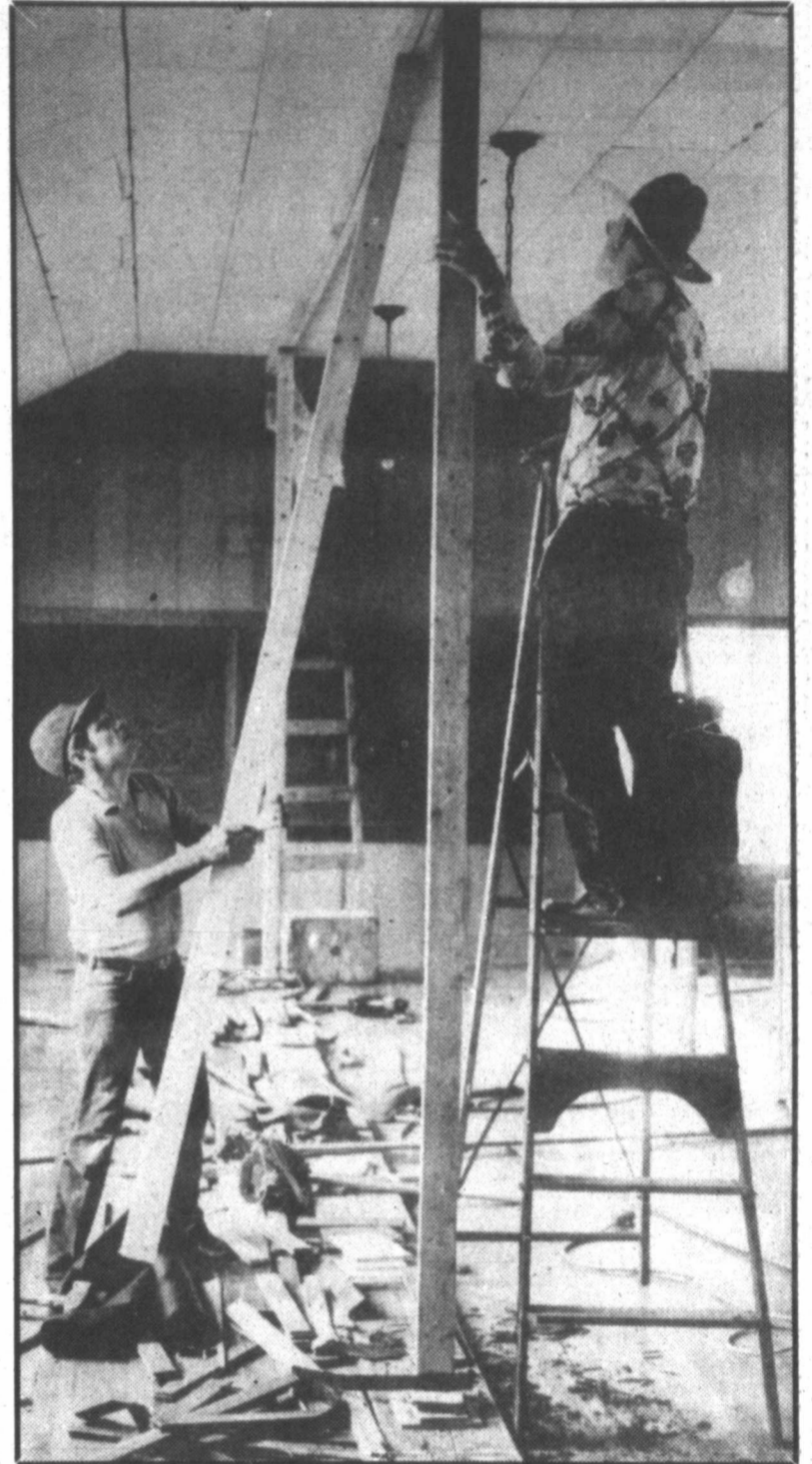
The Rev. Burd removes a support beam while fellow workers stand on ladders to steady the support brace.
