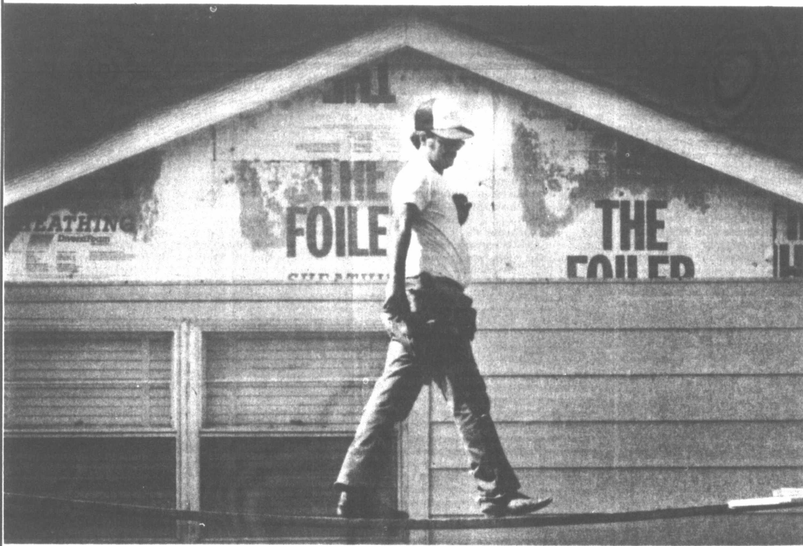
Jerry Anthony, an employee of John Anthony Construction of Pampa, walks steadily across a bending board while putting up siding on a residence on North Russell Street.
