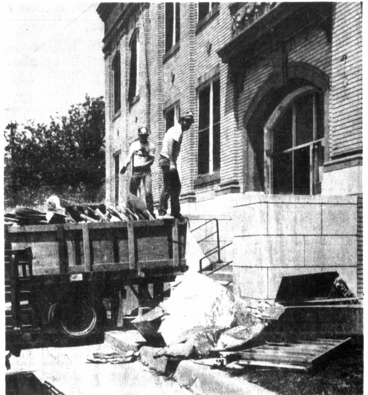
SO LONG, FAREWELL — Workers prepare to cart off another load of junk removed from City Hall during the city's renovation project. Renovation began last week. (Staff photo by Paul Pinkham.)
