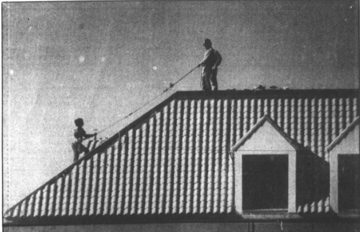
TILE MOUNTAIN — Like mountain climbers nearing a summit, workers are nearing completion of the roof of the new Corpus Christi Public Library. The building is expected to be completed in the spring. (AP Laserphoto)
