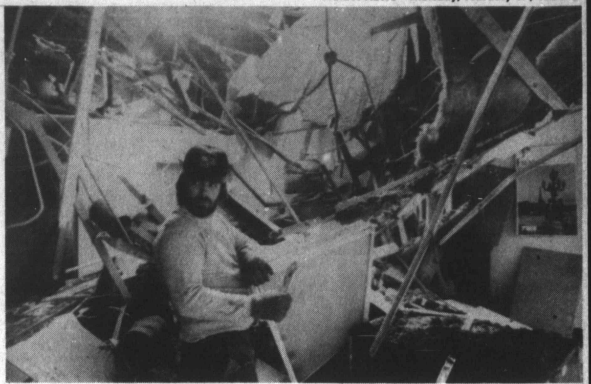
COLLAPSED BUSINESSES — James Jackson, an employee for a Salina, Kans., contractor, listens for instructions while disconnecting fixtures in Traylor Travel Service, located in downtown Salina. The building and two other businesses suffered major damage when the demolition of an adjacent
