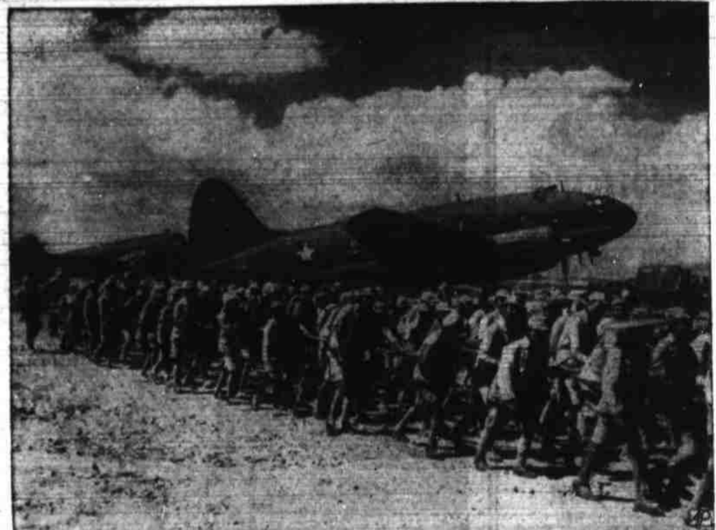
AIRPORT CONSTRUCTION —With a U. S. Army Curtis C-46 transport plane in the background, Chinese coolies and soldiers of an airfield garrison smooth runways at a Chinese airfield.
