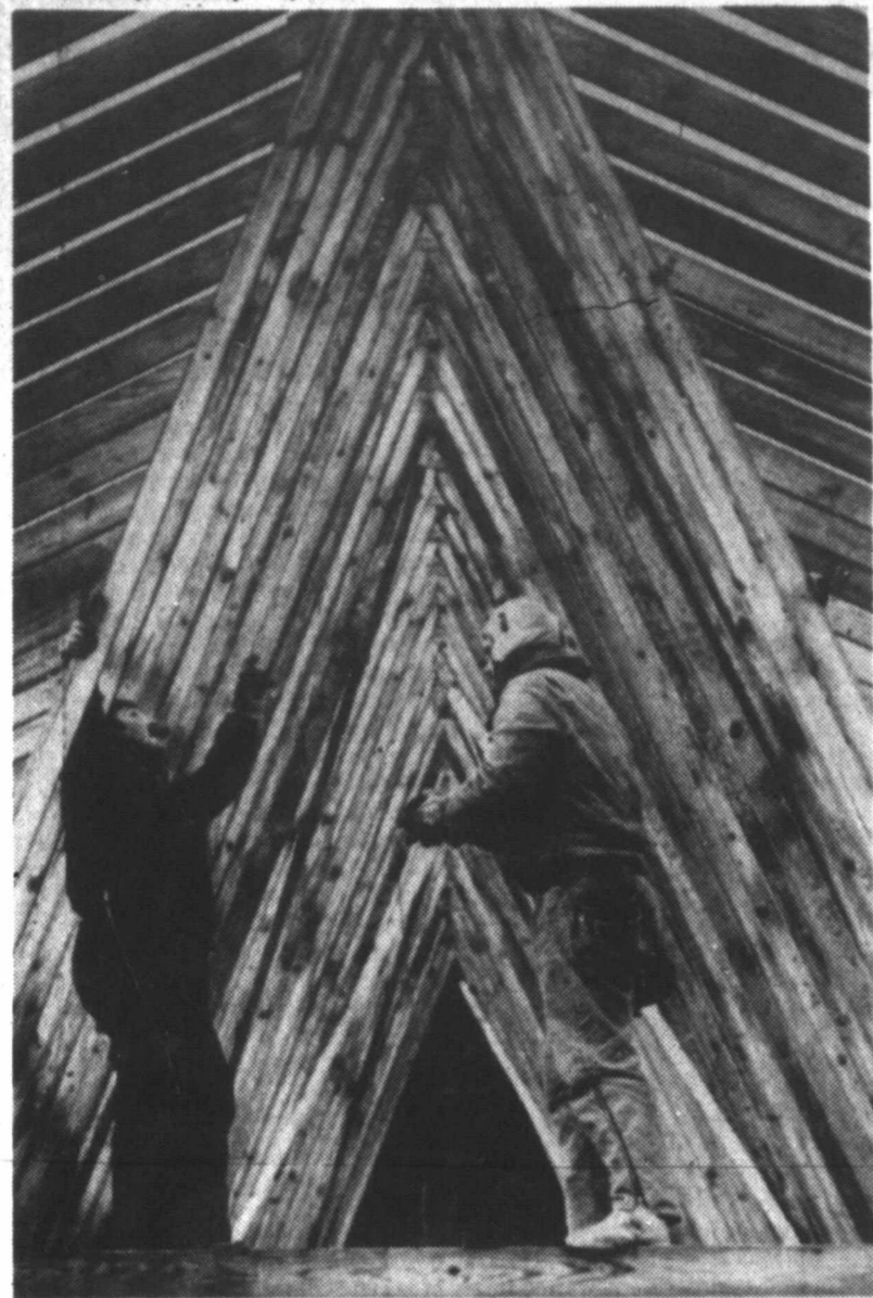
BOARD WALKERS — Clay Richardson, left, and Tommy Richmond take a break from their work on a new bank building in Palestine, Texas. The rafters make an interesting geometric pattern. (AP Laserphoto)
