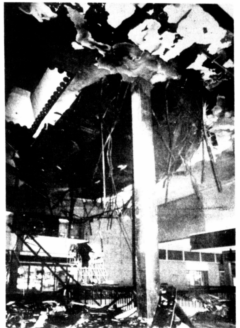
Plane knocks gaping hole in mall roof
