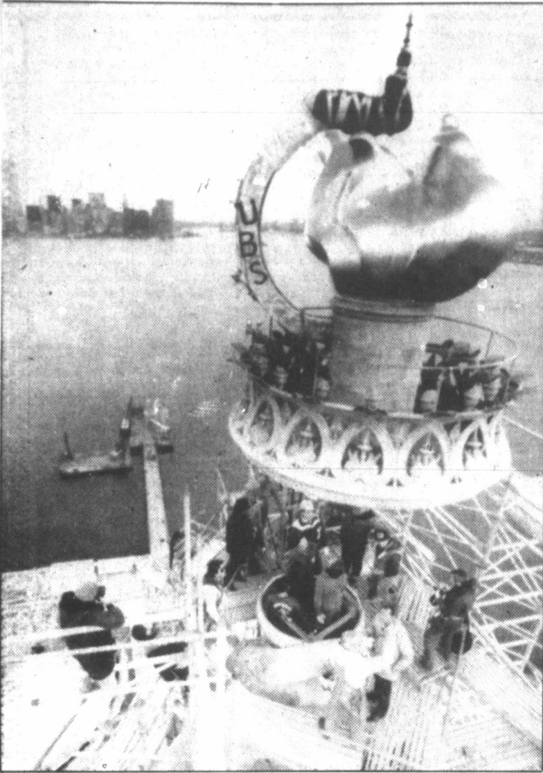
THE TORCH IS BACK — Workers guide the 2½-ton torch into place on the Statue of Liberty's upraised hand Monday, high above New York Harbor. About two dozen hardhats worked for two hours bolting a C-shaped hoist into the flame and balcony before raising the torch into place. The raising took 10 minutes. The flame is covered with several pounds of 24-karat gold leaf. (AP Laserphoto)
