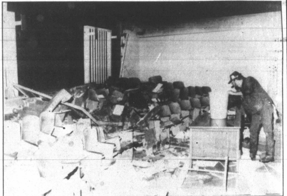
CLEANUP BEGINS — A worker removes debris from a classroom exposed to the elements following the collapse of a wall and the ripping off of the roof of a school in Broken Arrow, Okla., during a thunderstorm Wednesday. (AP Laserphoto)
