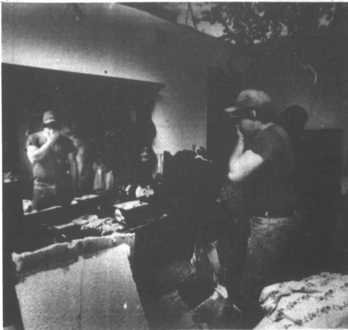
TORNADO AFTERMATH — Chris Grable wipes his eyes as he removes family belongings from the roofless bedroom of his parent's home near Dekalb, Mo. Several tornadoes swept through the towns of Agency, Faucett and Dekalb, south of St. Joseph, causing heavy damage Thursday evening. (AP Laserphoto)
