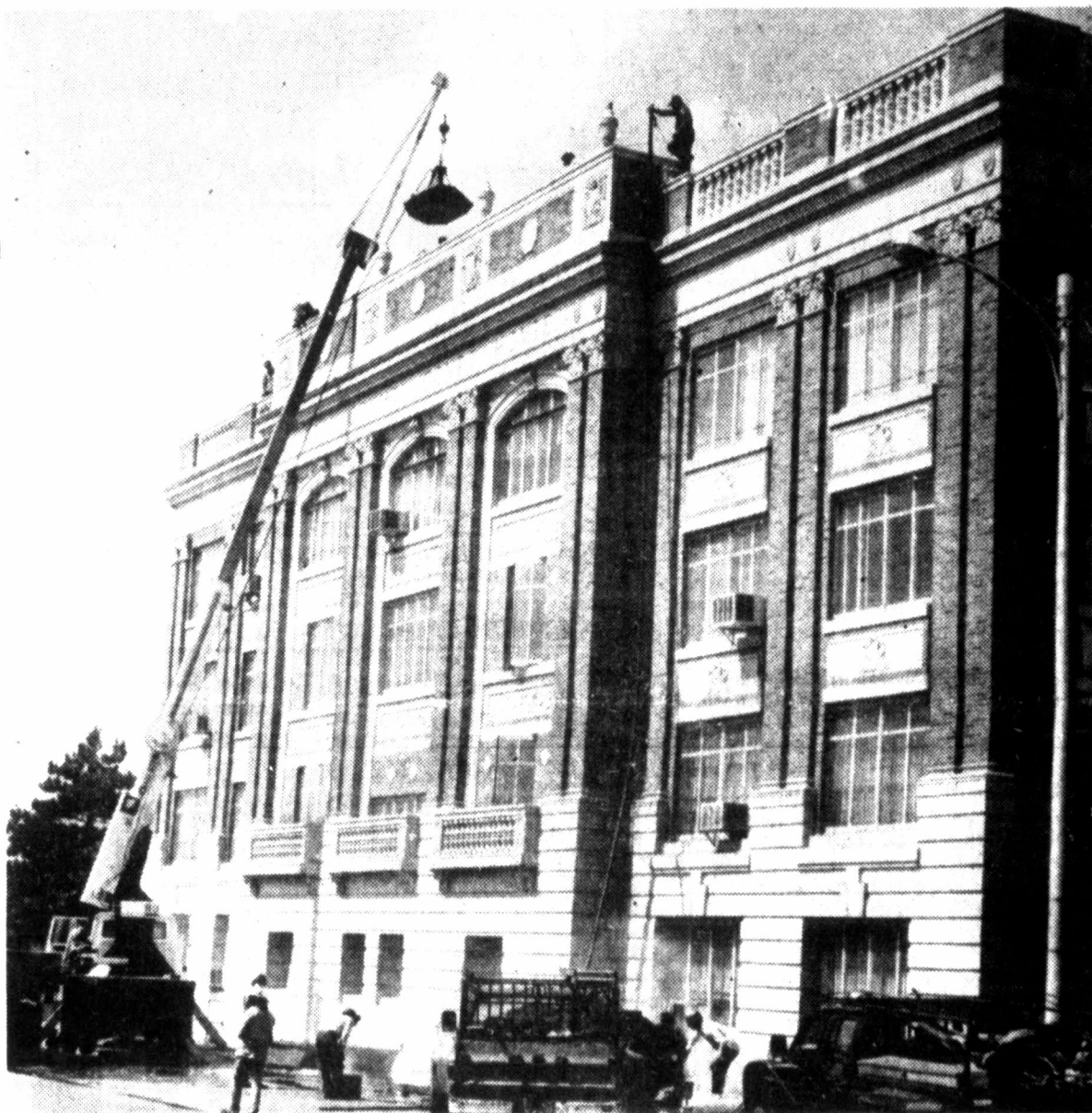
A TALL TASK — Workers from an area roofing company take advantage of Monday's Memorial Day holiday to repair the roof of the Gray County Courthouse. County Judge Carl Kennedy said that repairs to the courthouse,
