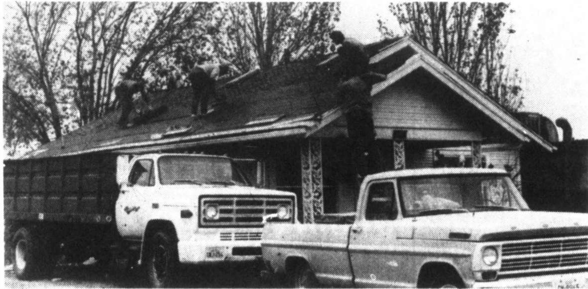
ROOF WORK—This group of Mennonite church members from Perryton have assisted the Red Cross in repairing hail-damaged roofs for about three weeks. But they have had to return home, creating a need for volunteer workers. (Staff photo by Revina Smith)
