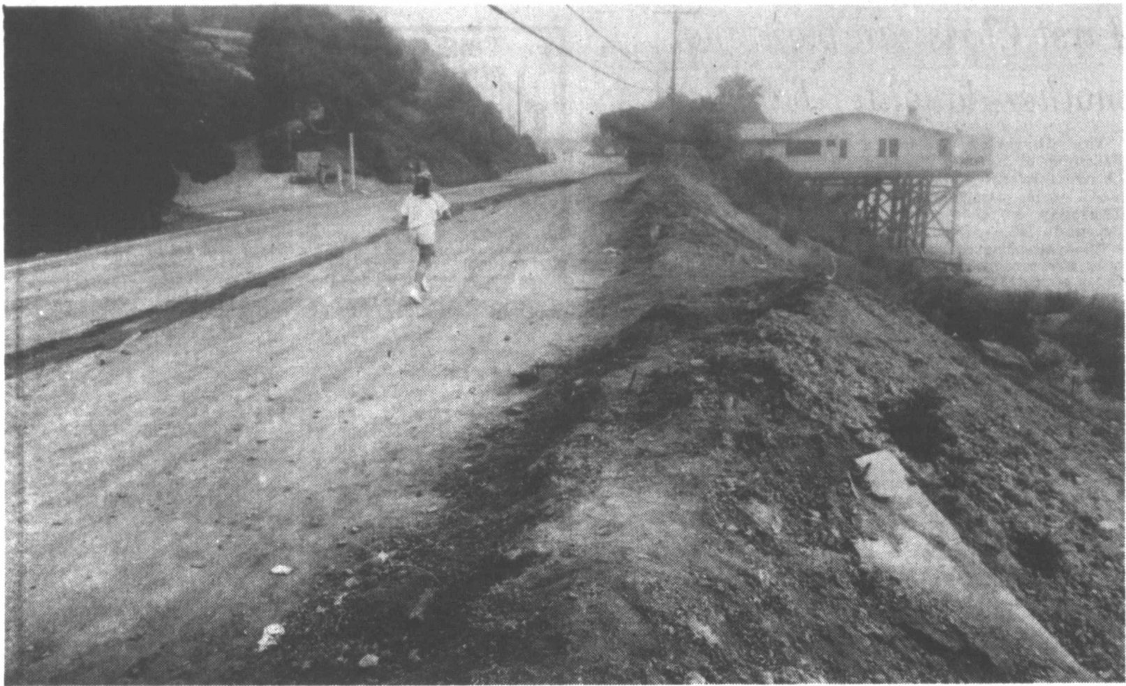
OLD MALIBU ROAD—A lone jogger runs along a deteriorating section of Old Malibu Road near Malibu, Calif.
