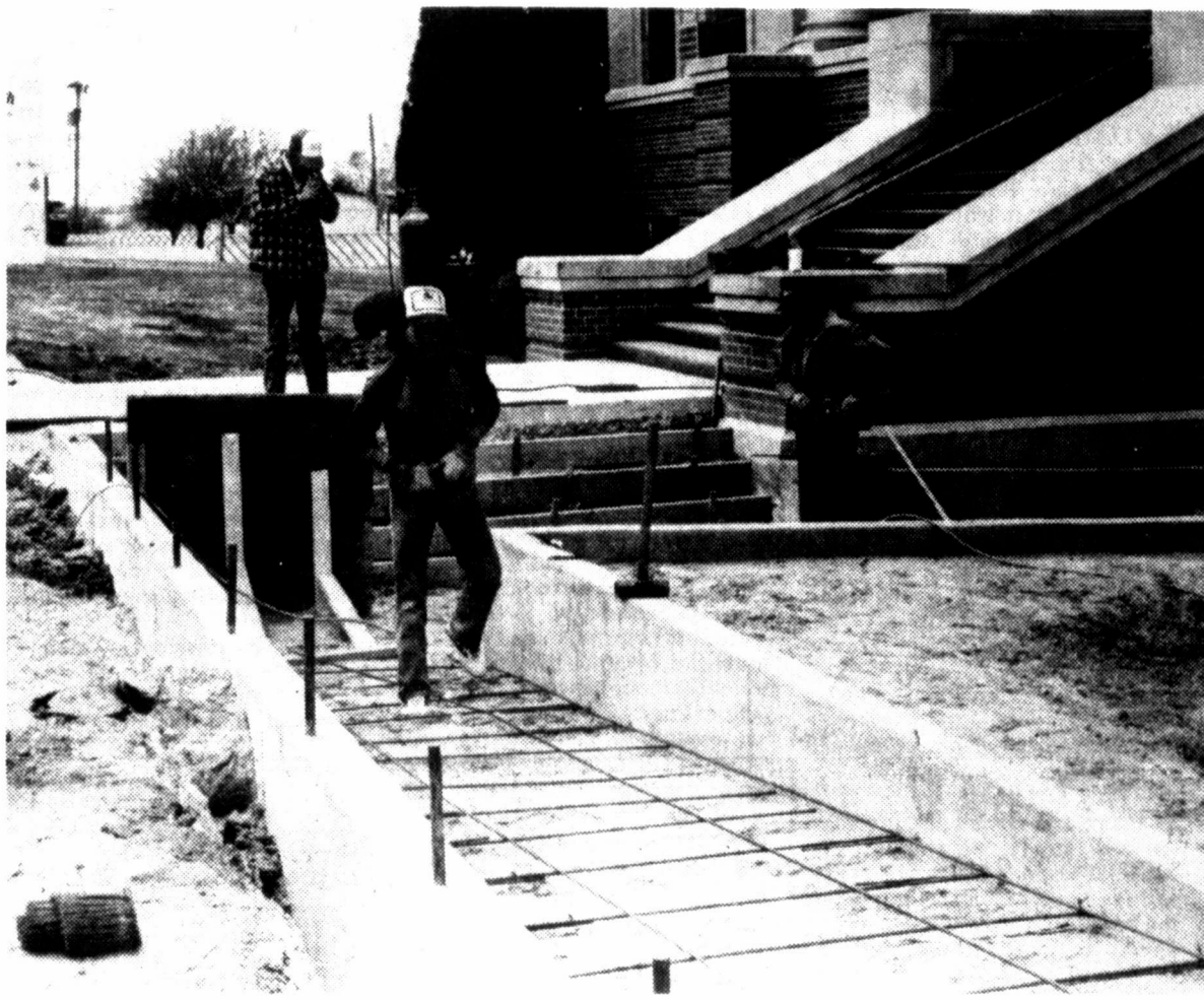
RAMP WORK — An employee with an Amarillo construction firm aligns steel reinforcement rods during construction of a wheelchair ramp and stairs at the Roberts County Courthouse.
